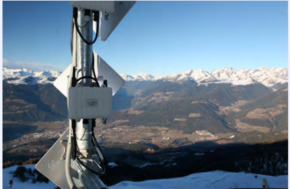
Celtic-Plus project CIER – Connecting the rural areas past the fiber-reach in the rural municipality of Bruneck / South Tyrol with WiBACK (Wireless Backhaul), developed in the Finnish-French; source: Fraunhofer FOKUS
