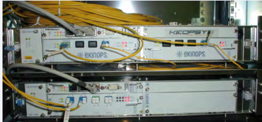
Figure 1: Receiver side and low-cost hybrid Raman-Erbium optical amplifier deployed in the field on the Lyon-Marseille-Lyon link
